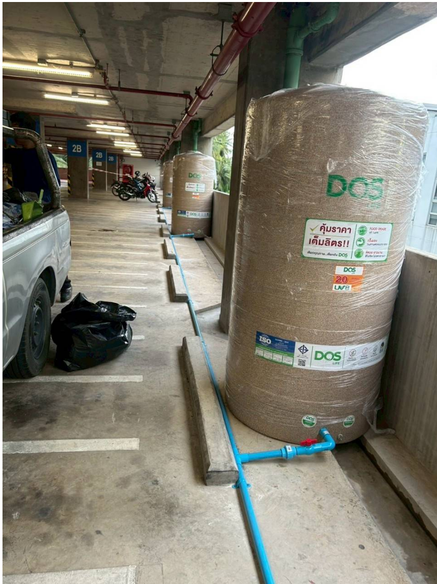
Rainwater Harvesting for Reuse
